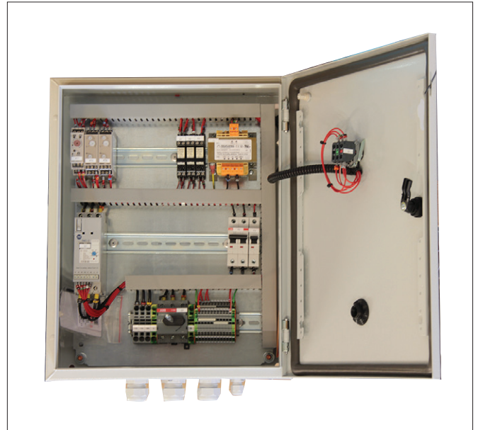
HVU Control panel
